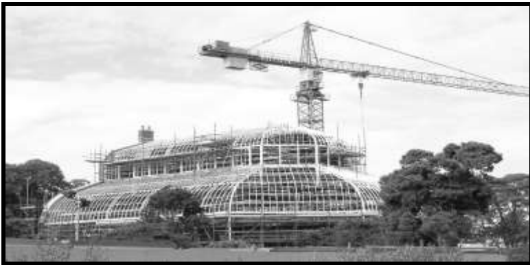
Work in progress on the Great Palm House, August 2003. Photo: P. Tobin
